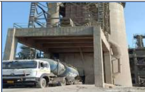
Fly ash transportation through bulker & unloading.
