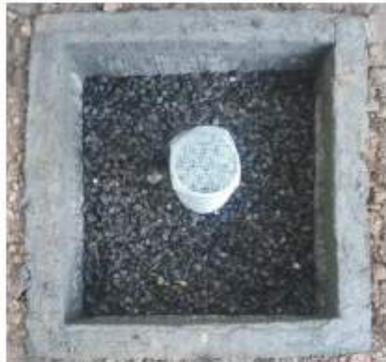
GROUND WATER RECHARGE SYSTEM AT GOP
